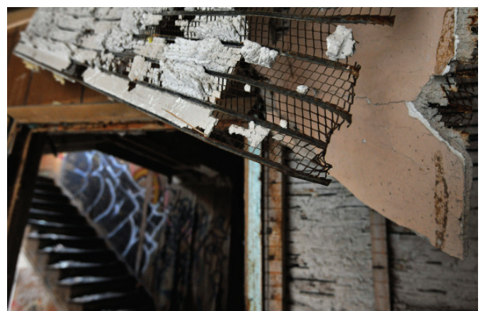
Interior crews could be confronted with the hazard of unstable walls, rotting roof structures, unprotected electricity connections and hazmat risks
